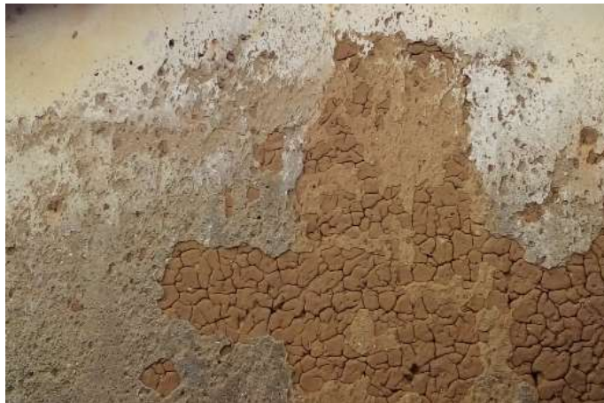
Figure 41. Picture showing how mud plaster and cement plaster don't bind together. Hence cement plaster comes off.
