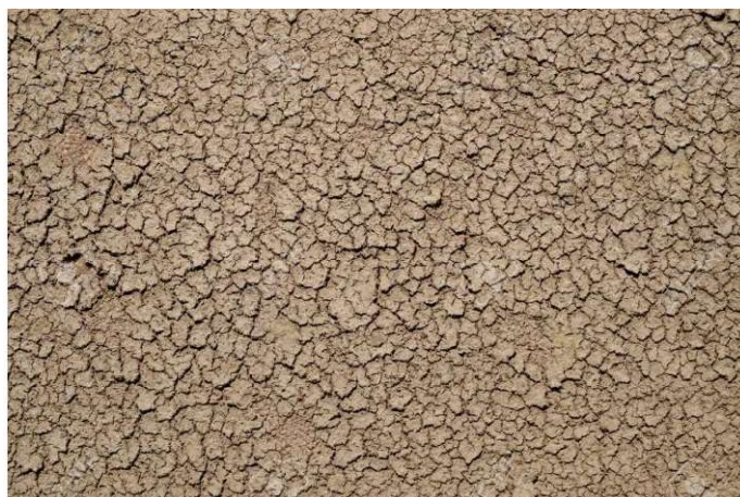
Figure 39. Example of poor quality mud plaster and mud constituent come off - to be avoided
