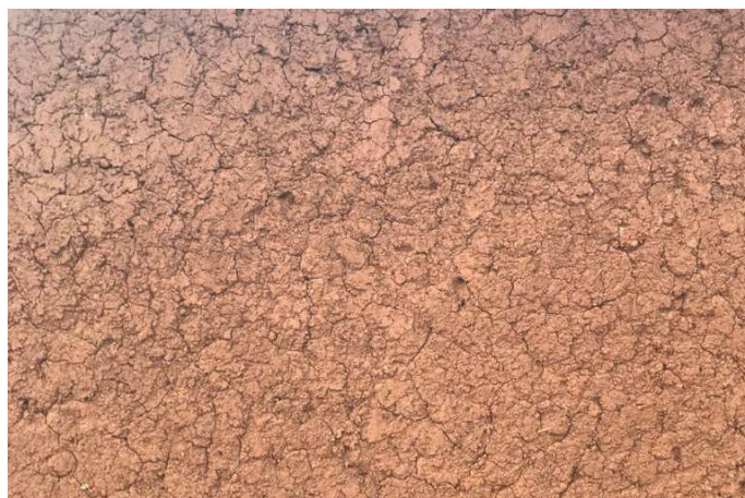
Figure 40. A good mud plaster has fewer cracks and mud constituent doesn't come off
